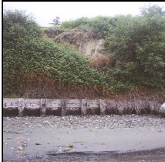
Figure 8: Structures are often intended to prevent erosion or to provide people with access to the shoreline. Both types of structures can negatively impact nearshore habitat, especially as the structures begin to fail.
