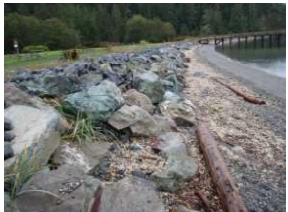
Project area before restoration including 540 linear feet and approximately 2,050 tons of rip rap armoring to be removed.
